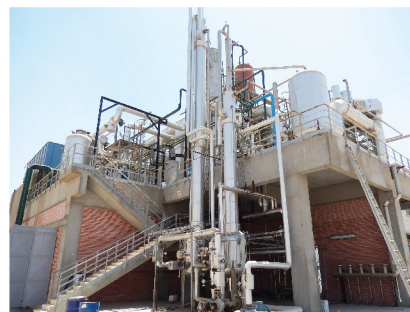
Plants for the recovery and reuse of solvents (Porta Egypt).
