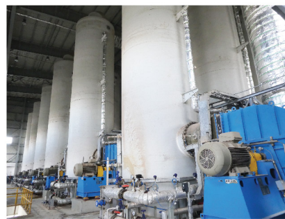
Wastewater treatment including stripping towers for ammonia recovery from wastewater to produce fertiliser (Abu Qir Fertilisers).
